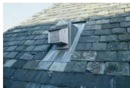
Bat box installed during the conversion of a school to offices at Norton Park, Edinburgh.
