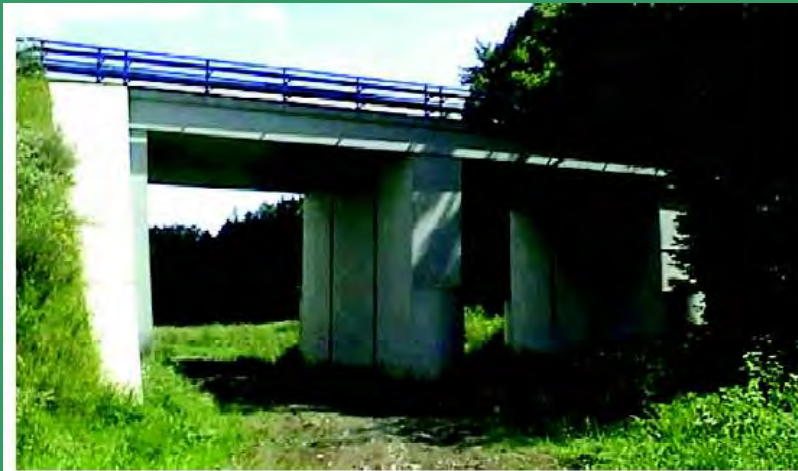
Figure 7.50 - An underpass below a railway line in the Czech Republic. It is combined with an agricultural track which is not tarmacked. Its height also makes it suitable for large mammals. (Photo by J. Dufek)
