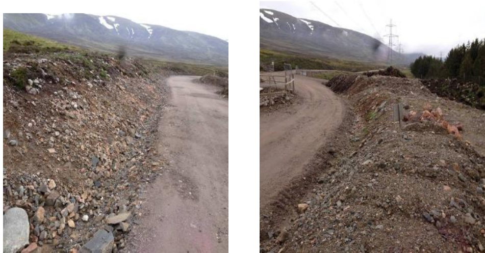
Figure 2: Photos of current cut and fill situation (Extract from Reinstatement Report for the Beauly Denny Line Access Track 25 – Ralia Estate)
