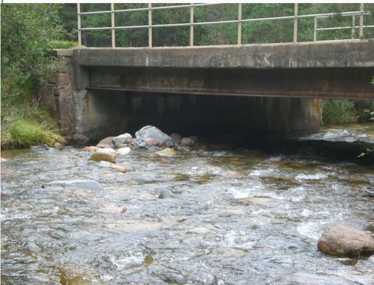
Allt Mhor bridge viewed from above. The flooding has created a new bank of boulders the opposite side of the bridge to that which was infilled last year. Photo credit Alan Bratney.
