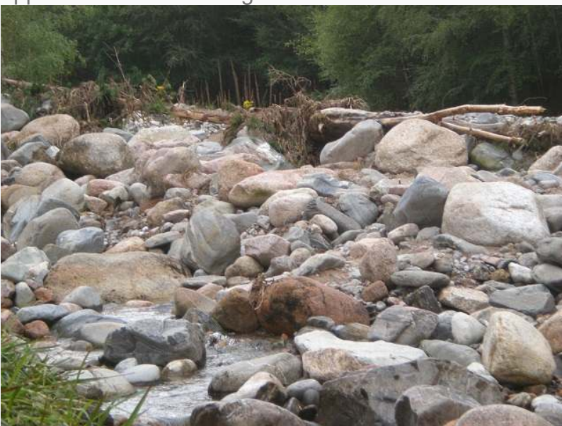
Just above the bridge are trees which, if washed against the bridge, could rapidly result in the channel under it blocking and the whole structure being swept away. Photo Credit Alan Bratney.
