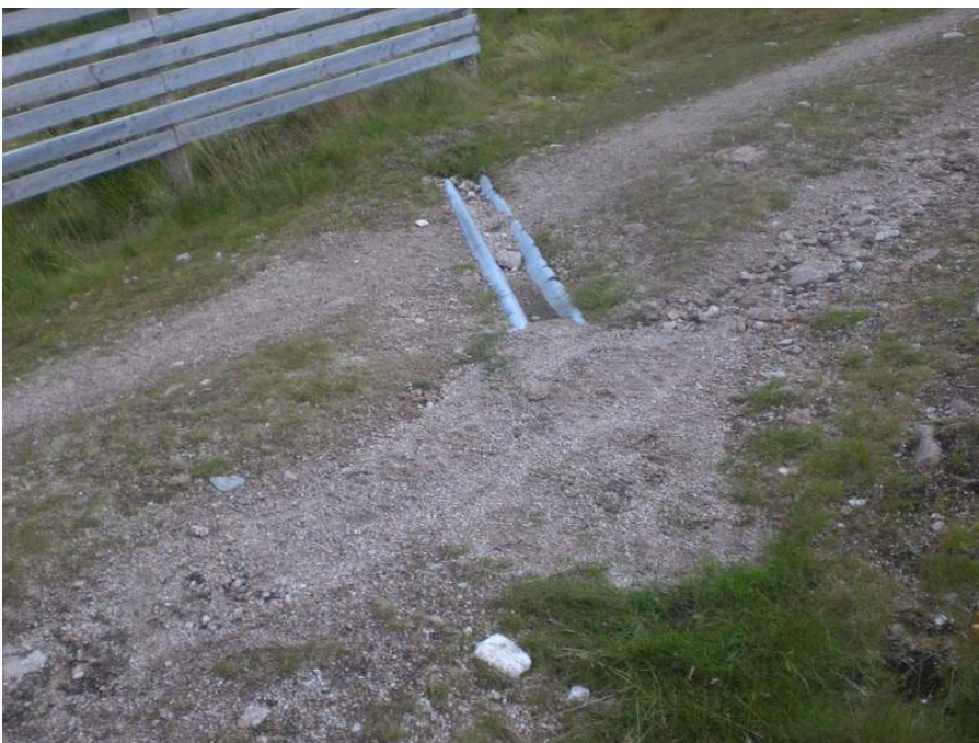
All the culverts below are still blocked and the consequences obvious. Photo Credit Alan Bratney.
