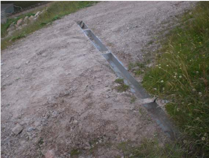
The top open culvert on the Shieling Rope tow track which has very recently been cleared of debris. Photo Credit Alan Bratney 24th August .
