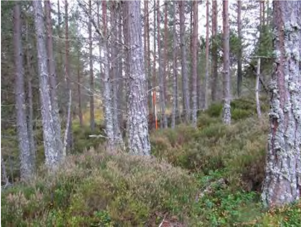
Bench cut ramp down to meet raised boardwalk position. Raised boardwalk for flood and All Abilities standards.
