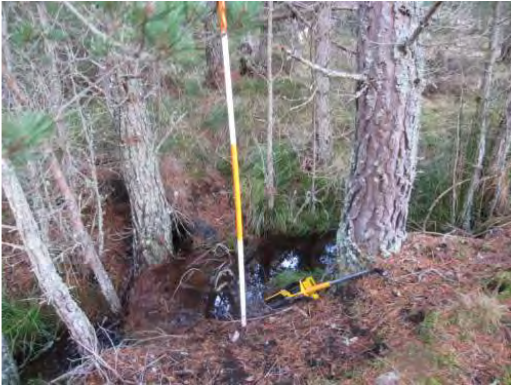
2no. 300mm culverts side by side with stone headwalls. Path angled between trees to keep width.
