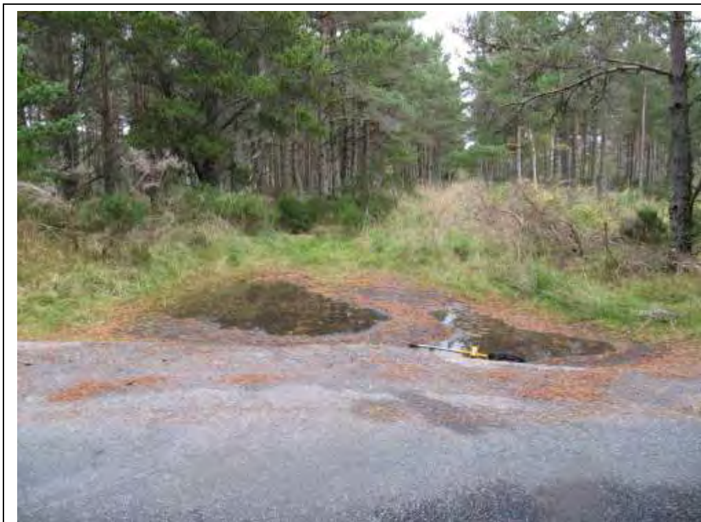
Splayed entrance to start of new all abilities path along start of old track to dump.
