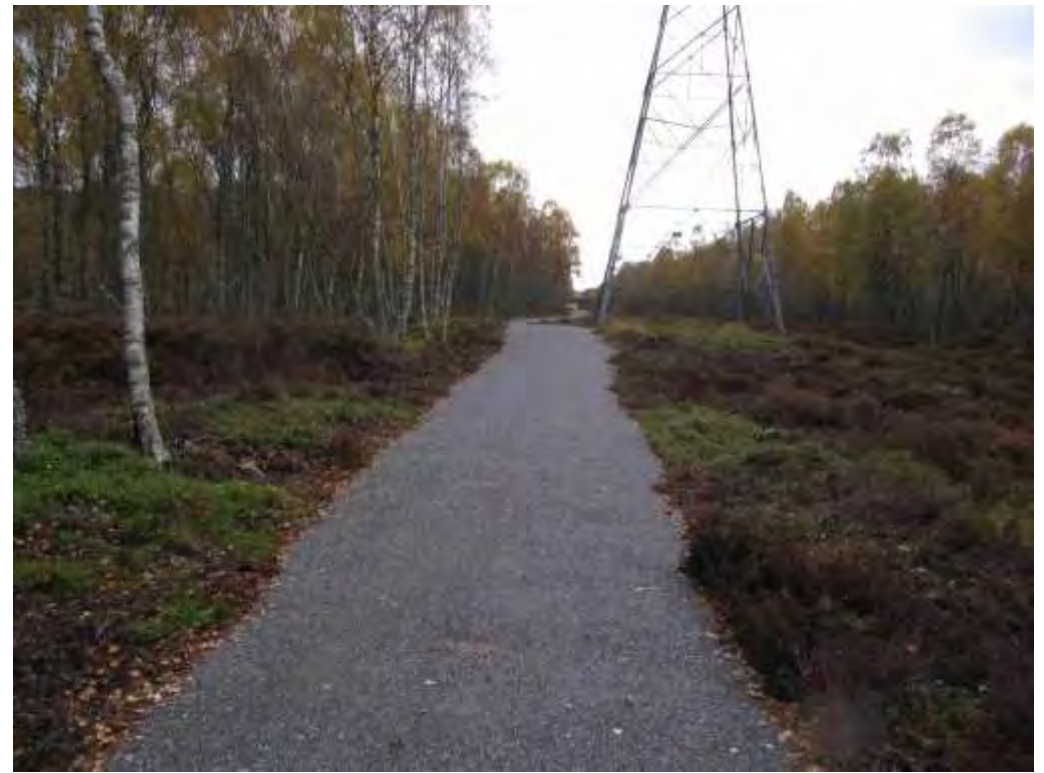
Example of recently constructed 'as dug' section of Speyside Way near Aviemore. 'As dug' ditches and borrow pits landscaped back in.
