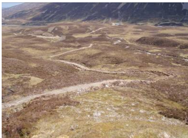
Fig. 3- View of works carried out, track in background is existing track to radio mast
