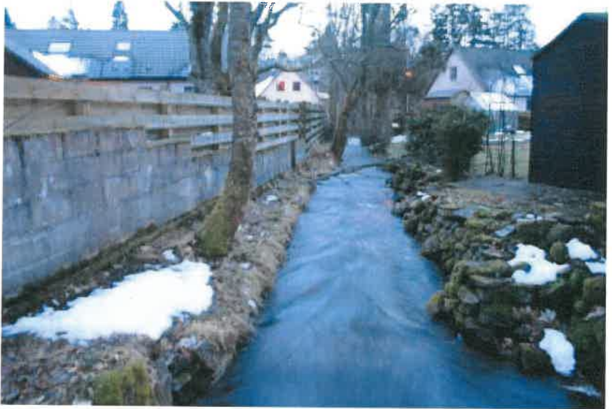
View of the 'canalised' section of the burn looking towards the Rhuarden Court culvert
