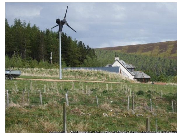
Figure 4 – free standing small scale turbine
