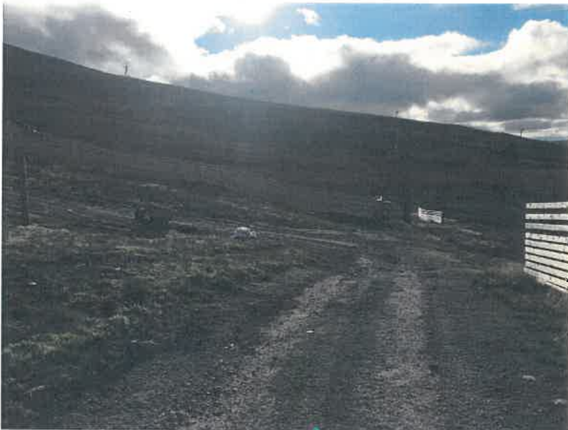
Image 7: Very small radius turn back up slope approaching top of the new Shelling Track.
