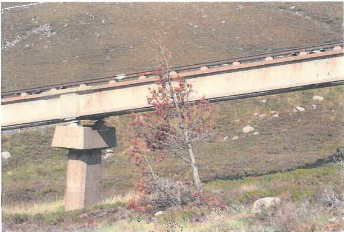
Image 1: One of numerous montaine scrub Scots Pines that has died post Sheiling Tow works due to combination of waterlogging and/or root damage through destruction of soil profiles and drainage creating an area of artificially boggy ground between new track and the Funicular.
