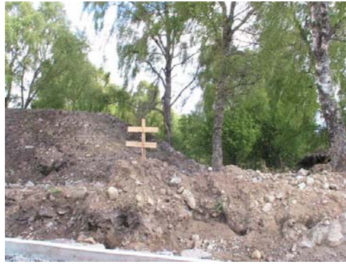
Fig. 19: Soil heaps in close proximity to trees in the western area of the site.
