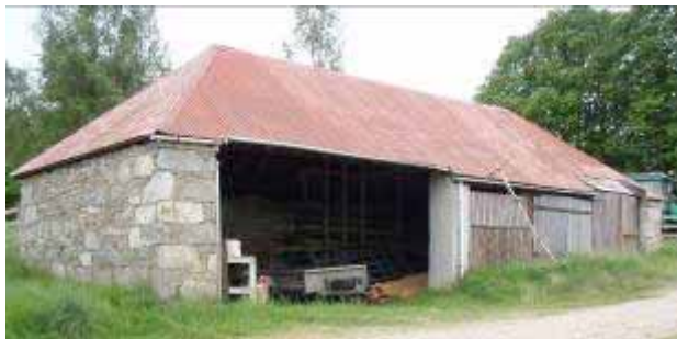
Fig. 11 : Existing tractor store which is proposed for conversion into 5 covered car parking bays
