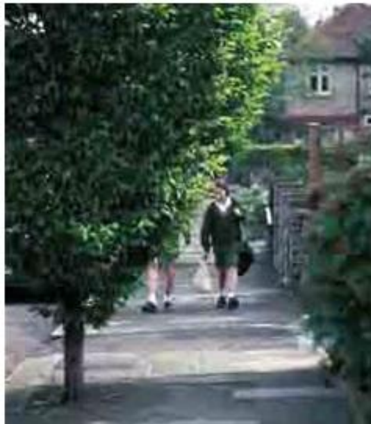
Figure G3.10 Poorly maintained tree obstructing the footway.
