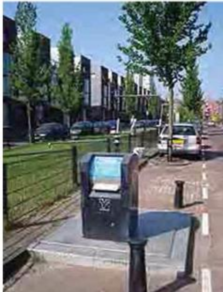
Figure G3.21 Refuse disposal point discharging into underground collection facility.
