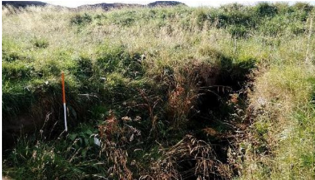
Figure 3.64 Culvert with erosion around the outlet at Drumgask Farm (OS NGR NN 61927 94037).
