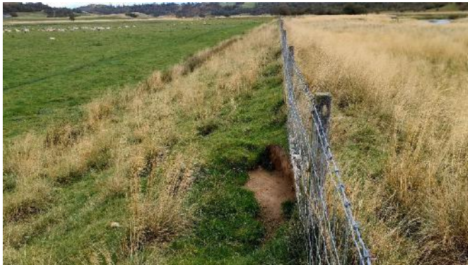
Figure 3.4 Low risk of embankment breach. Slumping of the embankment crest appears to have been caused by livestock trampling. The embankment is set back from the riverbank and signs of slumping observed are localised.
