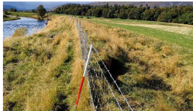
Figure 3.5 Moderate risk of embankment breach. Situated within 5 m of the riverbank, with slumping and bare ground exposed on the dry side of the embankment.
