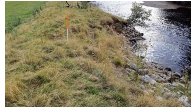
Figure 3.12 Riverbank erosion undermining an embankment positioned at the top of the bank. High risk of embankment breach.
