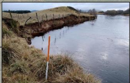
~40m long embankment breach.
