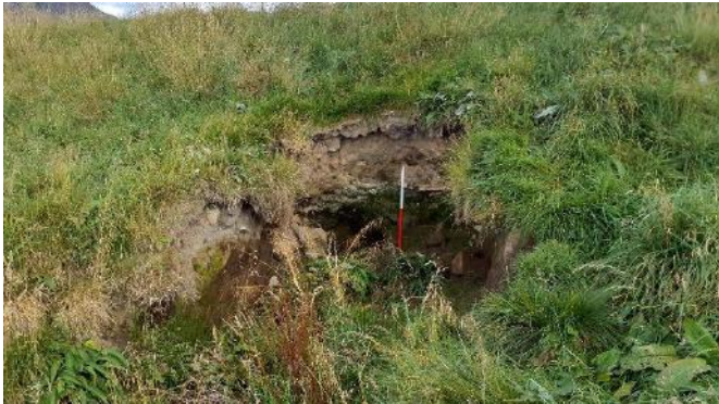
Figure 3.63 Culvert through the embankment with erosion around the inlet at Drumgask Farm (OS NGR NN 61927 94037).
