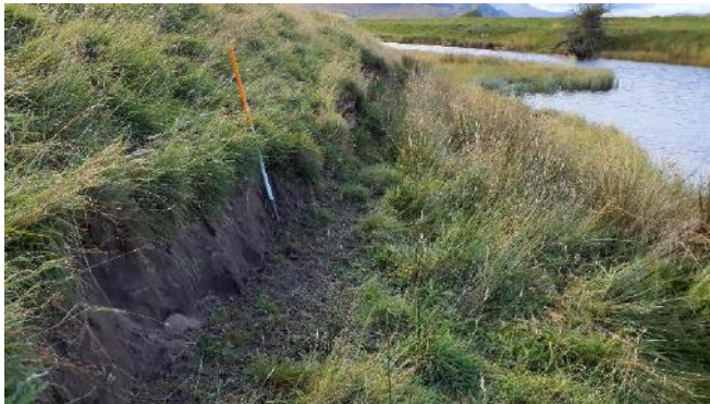
Figure 3.1. Low-severity riverbank erosion.
