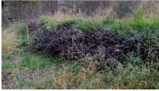
Figure 3.61 Example embankment breach remedial works. Large wood (trunks with root plates still attached) installed to protect the embankment face (OS NGR NH 88320 09028).
