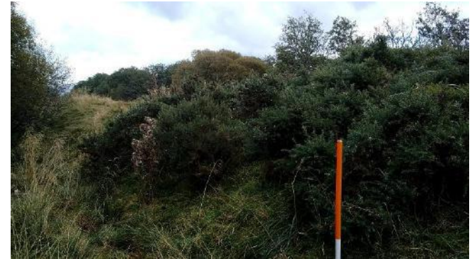
Figure 3.9. Scrub growth on the crest and face of an embankment.
