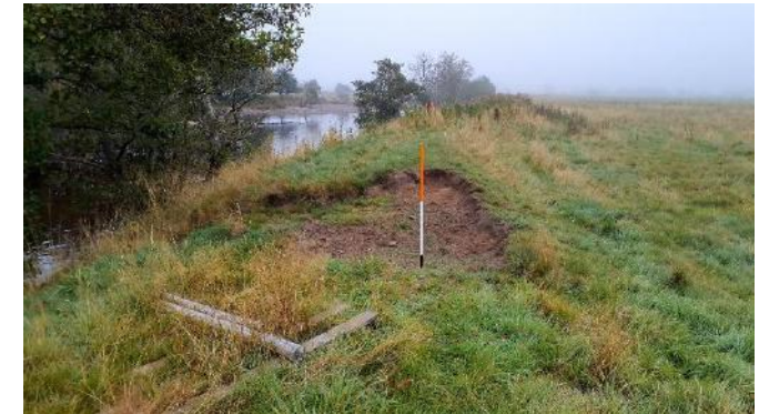
Figure 3.6 High risk of embankment breach. Embankment positioned along the top of the riverbank. Bare ground and slumping evident across over half of the embankment crest width.
