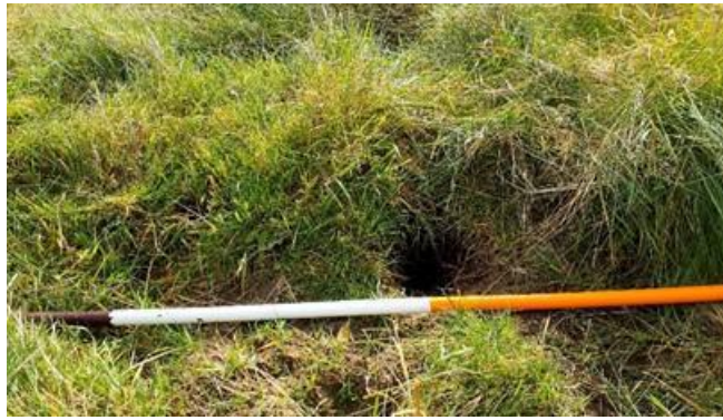
Figure 3.11 Burrow within the crest of an embankment. Mole hills and burrows were occasionally noted in Areas 1 and 2, but their position and density were insufficient to cause concern at the time of survey.
